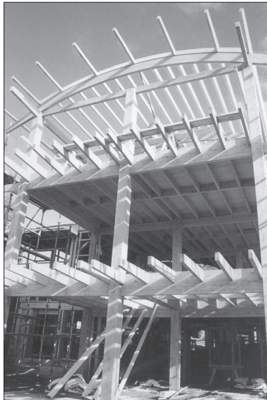
Three-story post and beam structure creates a unique feature demonstrating timber's natural strength and design possibilities.
